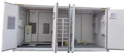
1075KW HH ESS
