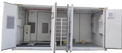
1075KW HH ESS
